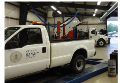
Veregy installed temp balancing destratification fans at the Fleet Building.
